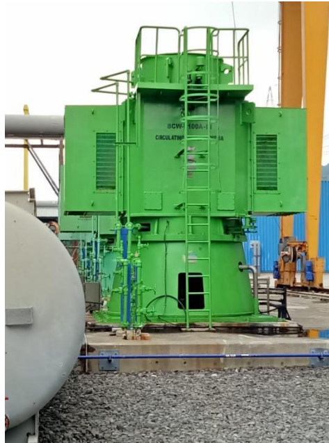
Gambar 3.16 Circulating Water Pump
