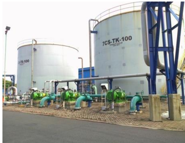
Gambar 3.21 Condensat Storage Tank Unit 5 & 6
