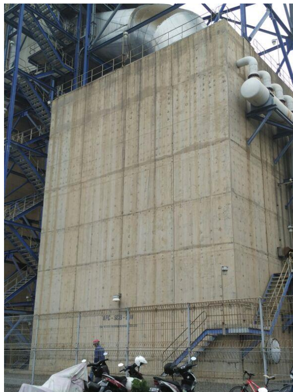
Gambar 3.32 Flue Gas Desulfurization (FGD)
