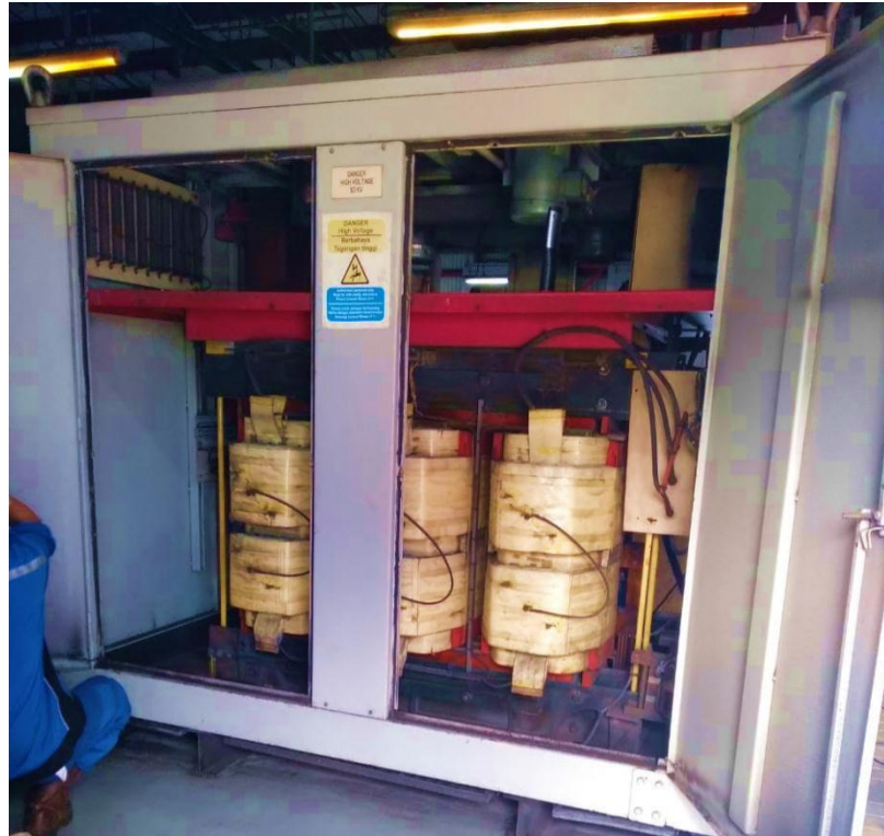
Gambar 5. 2 Dry Transformor (Step-down) 00BJT17
