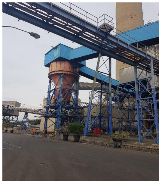
Gambar 3.34 Bottom Ash Silo
