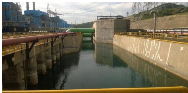
Gambar 3.15 Sea Water Intake
