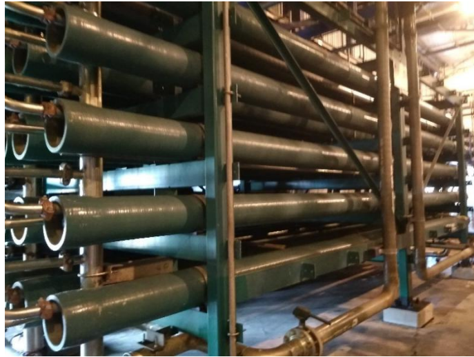
Gambar 3.17 Sea Water Reverse Osmosis (SWRO)
