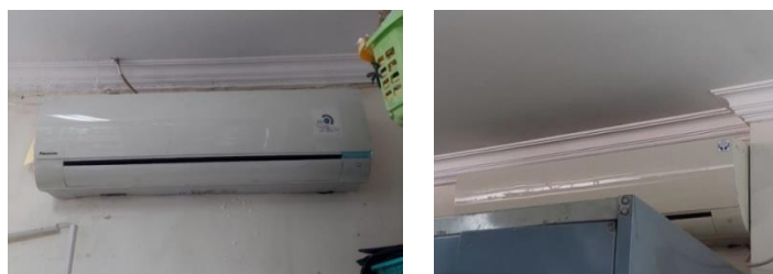
Gambar 1.4 Air Conditioner ruang filing atas
