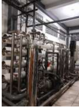
Gambar 3. 5 Mesin Reserve Osmosis (RO)
