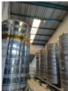
Gambar 3. 4 Tandon Final Tank
