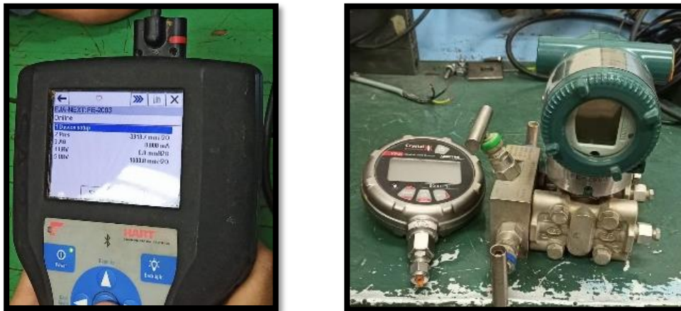
Gambar 14. Kalibrasi Transmitter (Differential Pressure)
