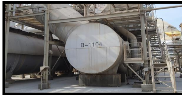
Gambar 19. Waste Heat Boiler
