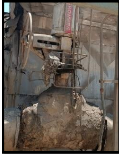
Gambar 38. TCV ( Temperature Control Valve )
