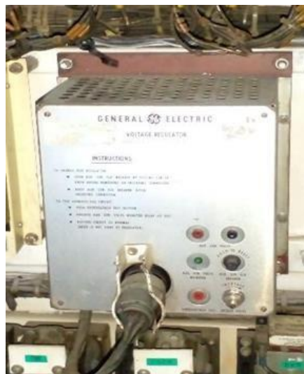
Gambar 3. 5 Automatic Voltage Regulator.
