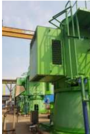
Gambar 4. 9 Circulating Water Pump
