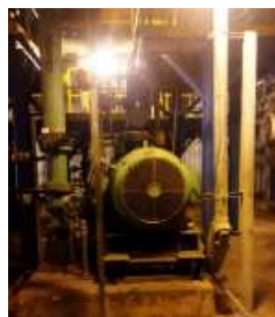
Gambar 4. 10 Vacum Pump Kondensor
