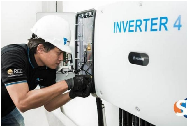
Gambar 4.3 Inverter Panel Surya
