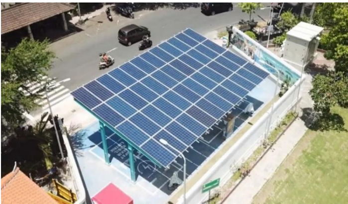
Gambar 3.4 Panel Surya Canopy
