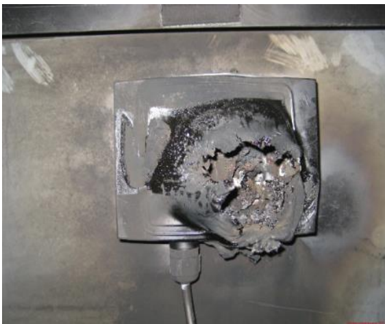
Gambar 5.18 Sirkuit Junction Box Terbuka (Sumber: ica solar)
