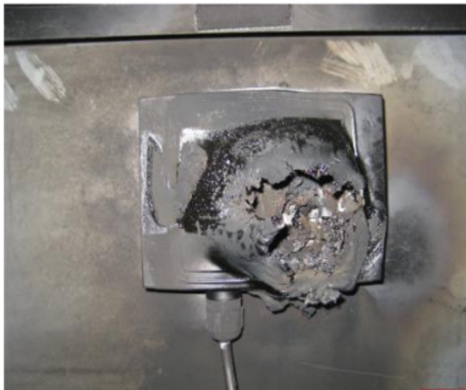
Gambar 5.18 Sirkuit Junction Box Terbuka (Sumber: ica solar)
