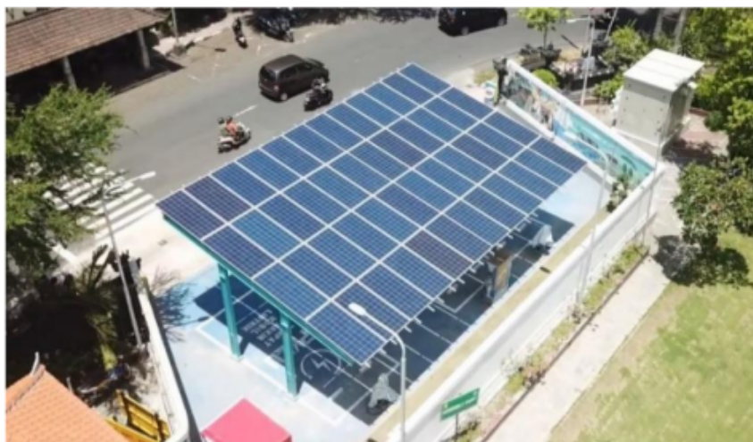
Gambar 3.4 Panel Surya Canopy
