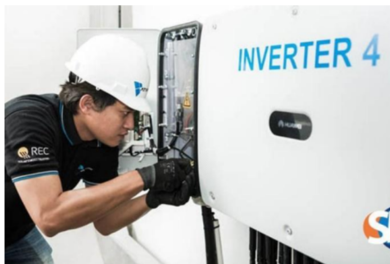
Gambar 4.3 Inverter Panel Surya
