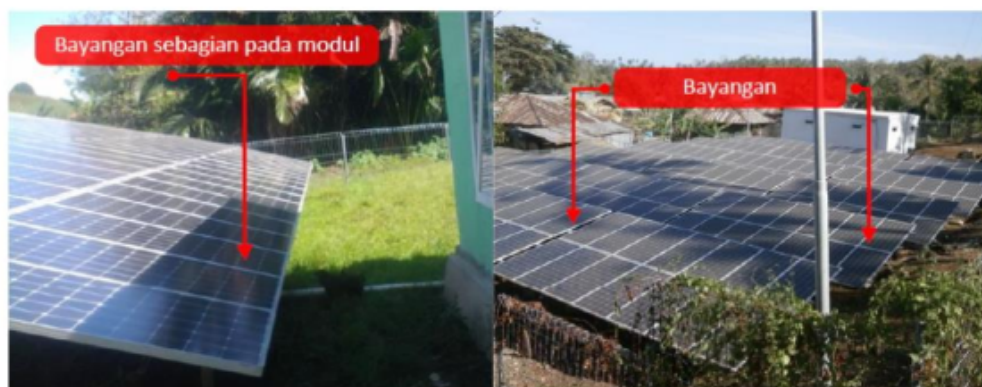
Gambar 5.14 Panel Surya Terkena Bayangan (Sumber: pasangpanelsurya.com)
