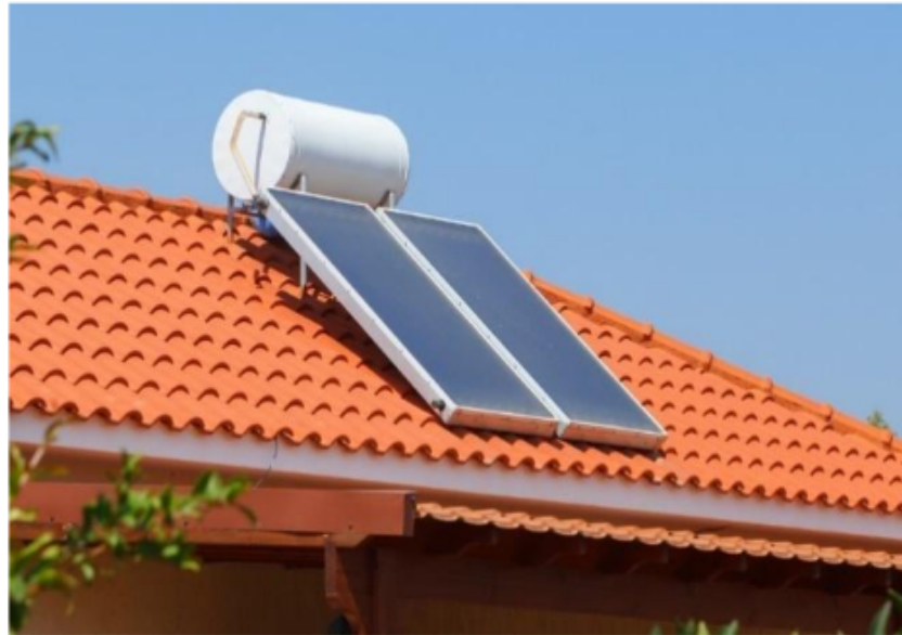
Gambar 3.5 Solar Water Heaters
