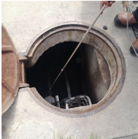
Gambar 3.18 Lifting Station (Sumber: Dokumen Pribadi,2022)
