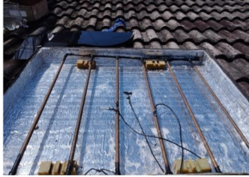
Figure 2. Copper pipe with evaporator chamber.
