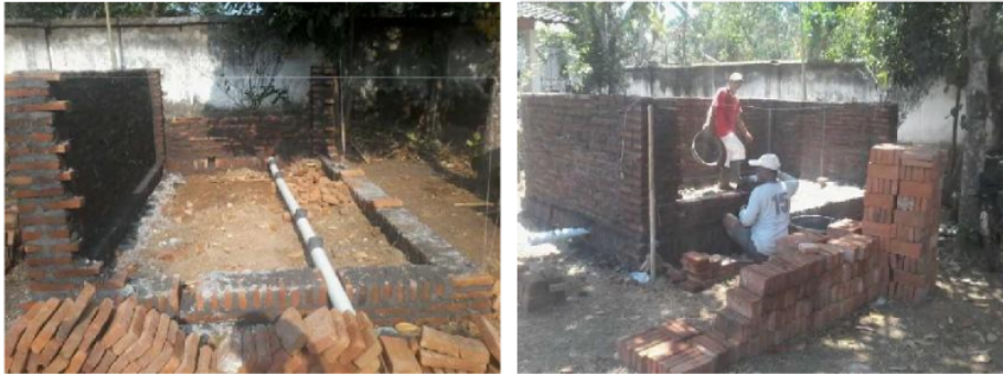
Figure 4. Material recovery facility for waste processing
