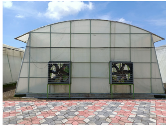
Fig. 20 Exhaust fan for effective circulation of the air in the smart green house
