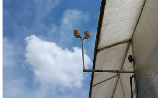
Fig. 19 Humidity and outdoor sensors determine the temperature difference inside and outside the smart green house
