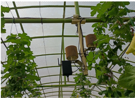
Fig. 18 Strategic placing of humidity and temperature sensors
