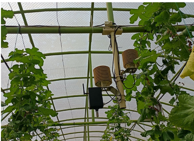
Fig. 18 Strategic placing of humidity and temperature sensors
