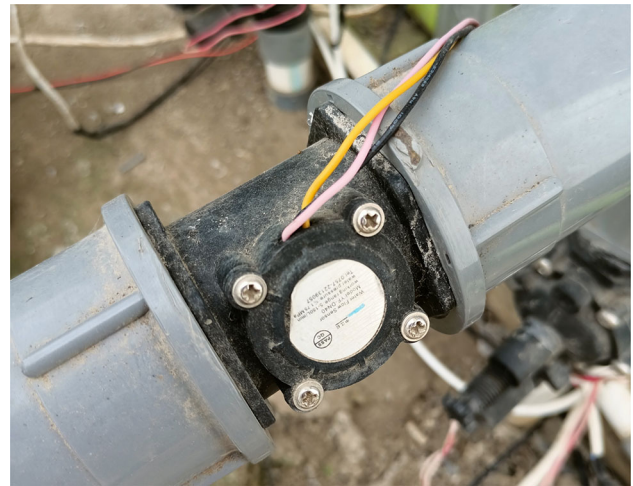
Fig. 12 Water flow sensor to calculate the plant's water discharge
