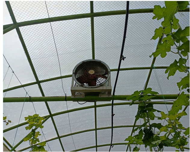
Fig. 22 A fan to circulate the air within the smart green house
