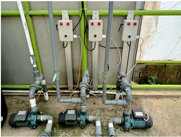
Fig. 13 Misting pump control, nutrition and irrigation, cooling deck
