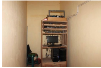
Gambar 2. Survey Kesiapan Ruang Server Internet
